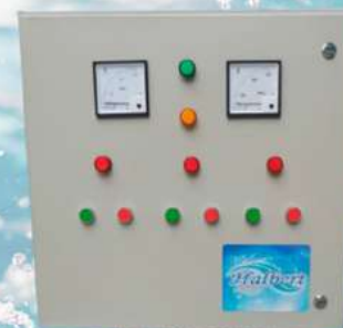
Electrical Control Panel
